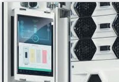
Measure and control energy consumption
