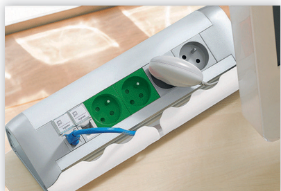
Supplying power to workstations
