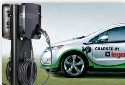
Electric vehicle charging
